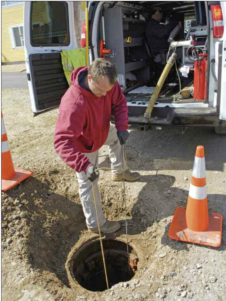
Keith Emory lowers an Envirosight camera and robotic crawler into a sewer line during an inspection.
